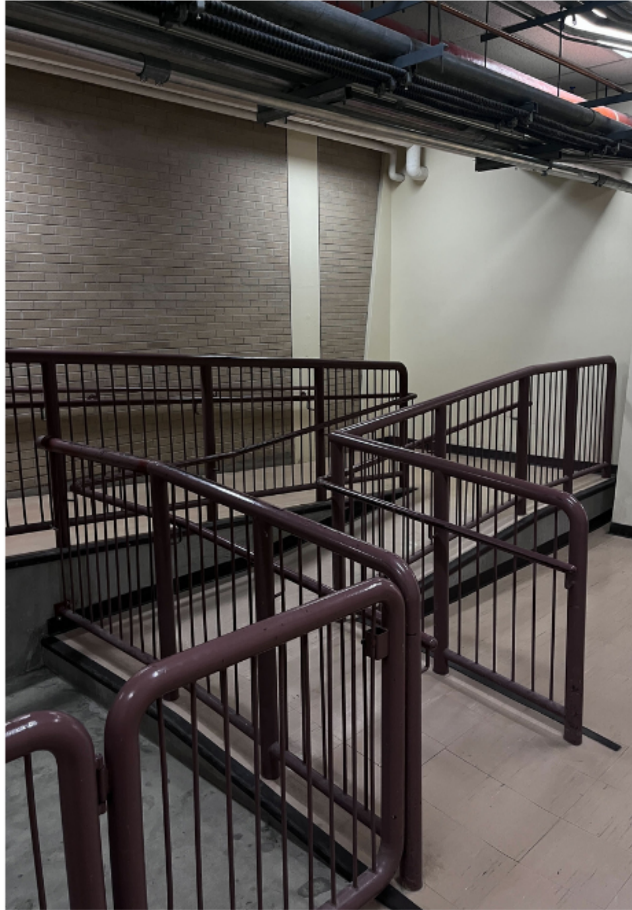
Accessibility ramp connecting the arts tunnel to Edwards | Francisca Lopez Molina, The Sheaf
